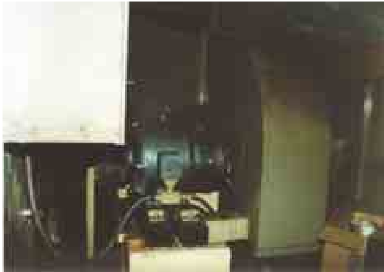
Fig. 37 Air conditioning plant
