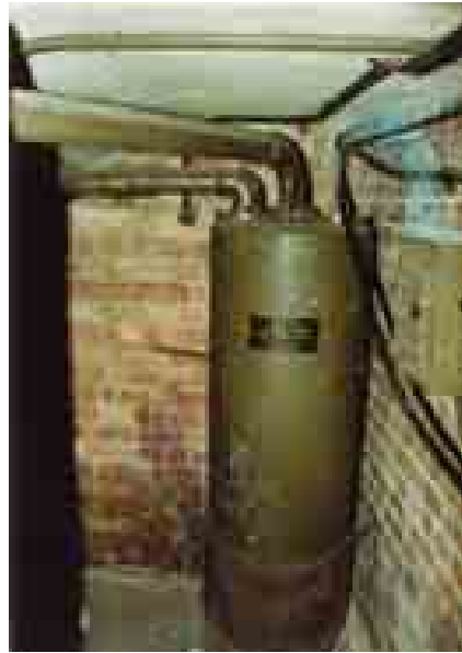
Fig. 40 The BVC centralised vacuum cleaner plant
