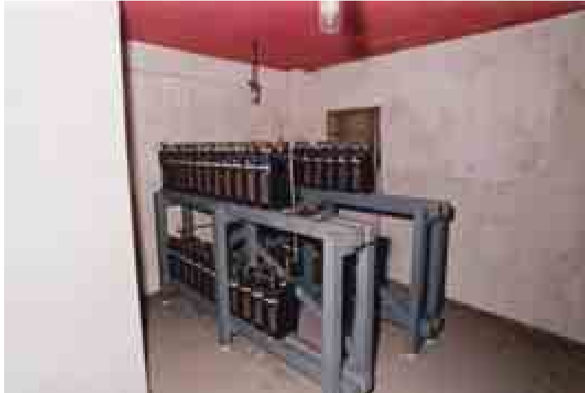
Fig. 18 Emergency lighting battery
