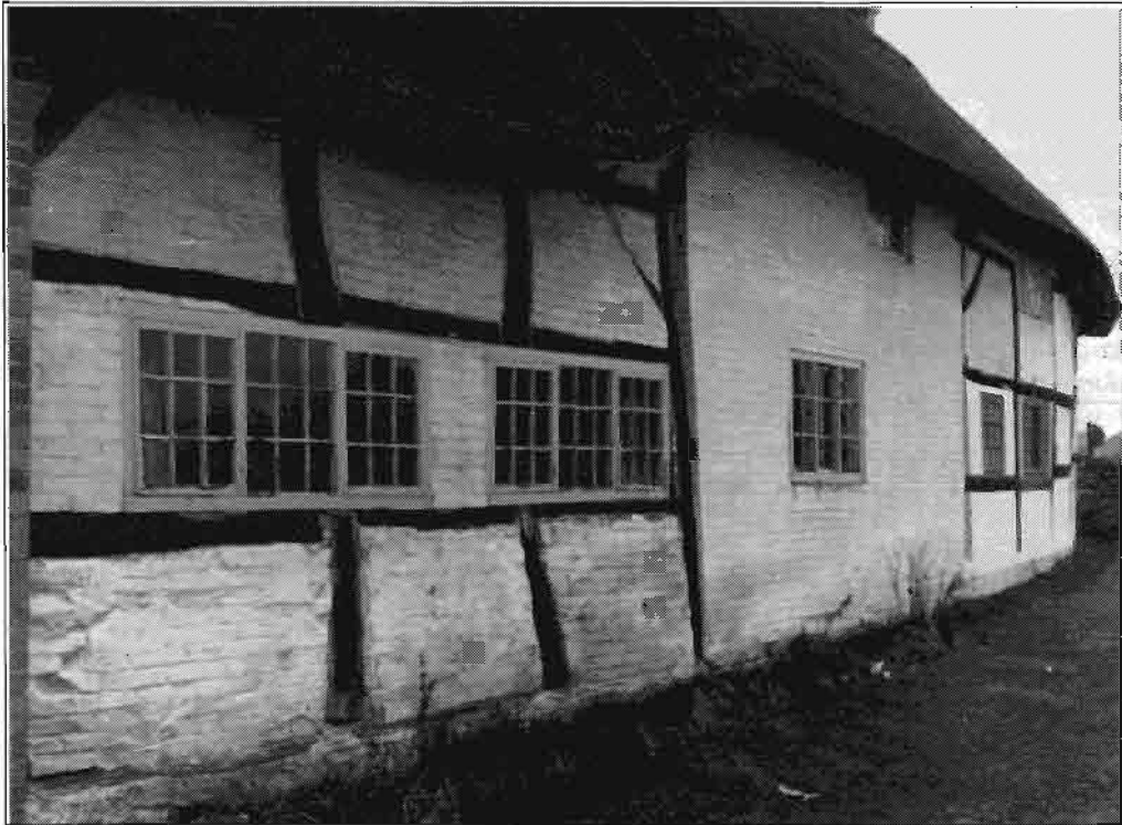
2. A timber- framed house in Shepshed, showing the extension containing long windows which have been inserted by cutting through the timber framing.
