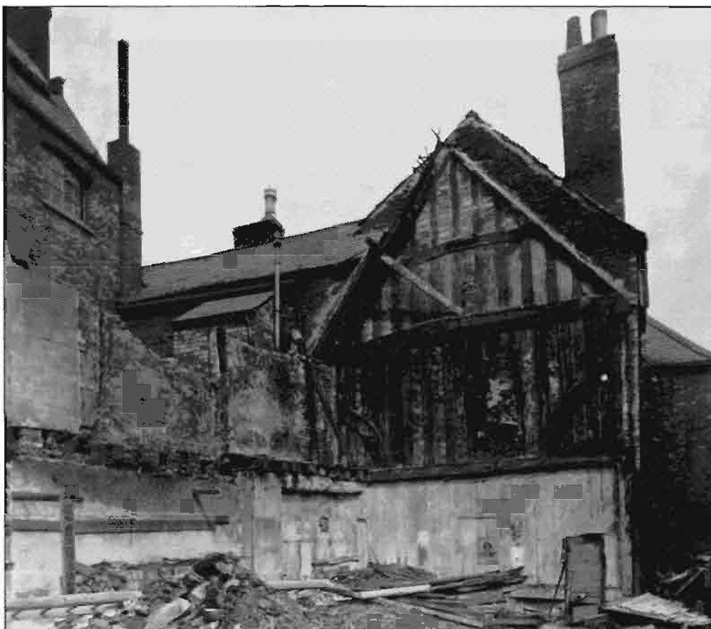
6. Timber framed building at rear of tower during demolition, viewed from south
