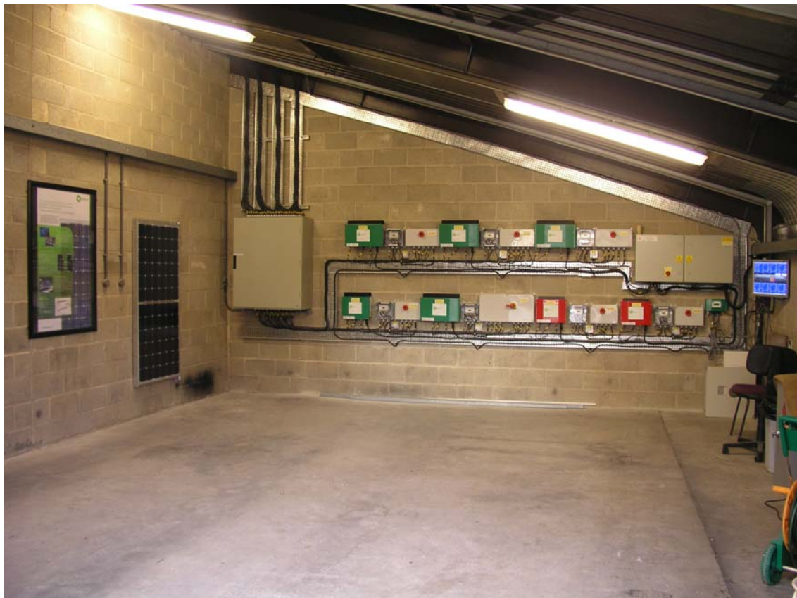
Photo 3 Electrical installation inside Concrete Laboratory
