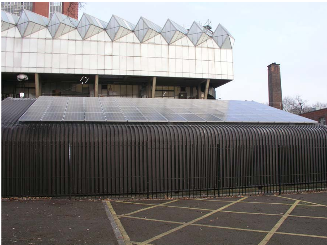
Photo 1 PV array on roof of the Concrete Laboratory
